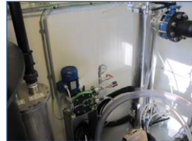
Figure 6: Inner view of container with substrate tank to the left, substrate feed pump in the middle and filter column to the right
